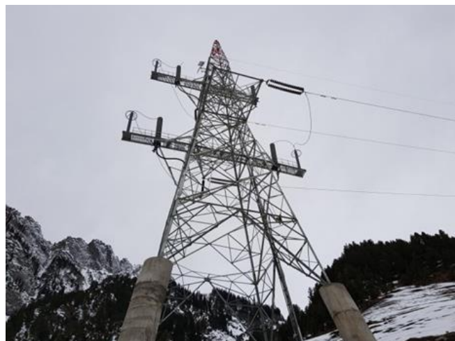
220kV S/C Cable Termination Tower at Sonmarg (J&K)
