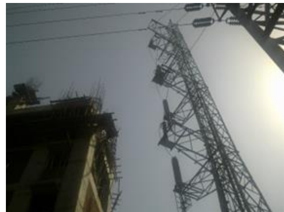
220kV Multi-ckt. /Multi voltage cable termination at Goregaon(W) Mumbai
