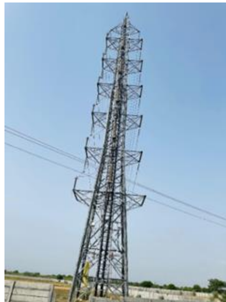
220kV M/C Cable Termination Tower, Ahmedabad
