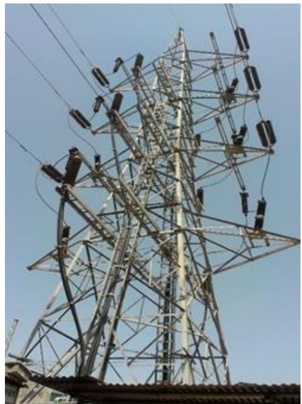
132kV Cable Termination
